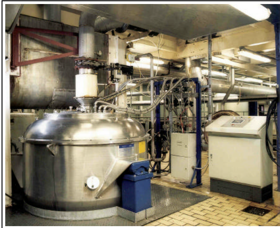
.Fig 2. View of High Grade Continuous Centrifugal installation in Europe.
